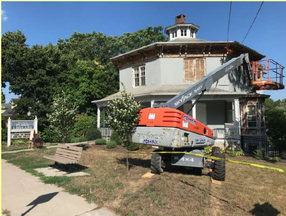
In 2020 grants and donations made it possible to scrape, repair, and apply fresh paint to the octagon's 155 year old wooden trim.
